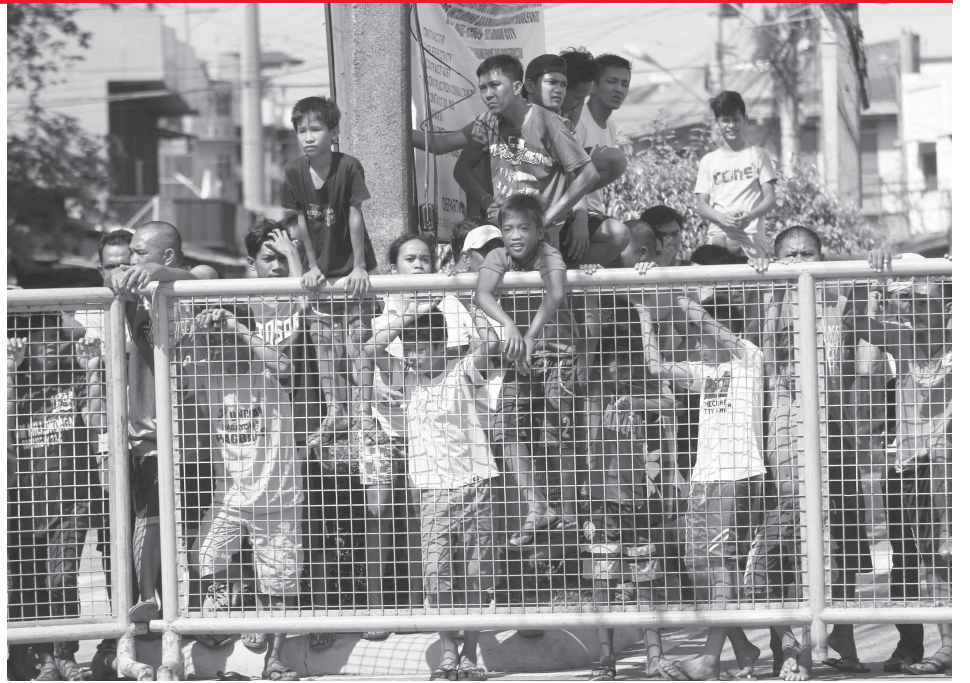
Residents of nearby barangay watch behind metal barriers while concrete houses and shanties are being demolished in Brgy. 26-C Salmonan, Quezon Boulevard on Monday. Lean Daval Jr
